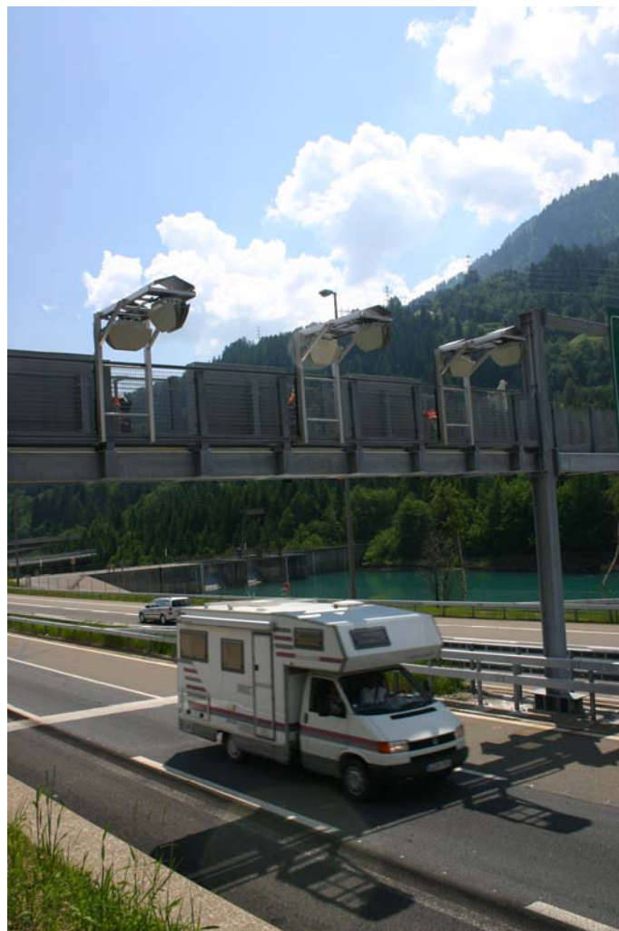
TIC System in Airolo on the south side of the Gotthard tunnel
